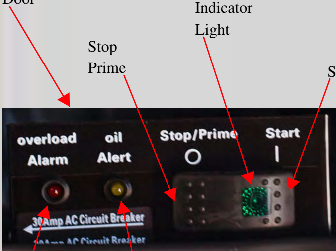
Start/Stop Switch inside Generator Service Access Door
